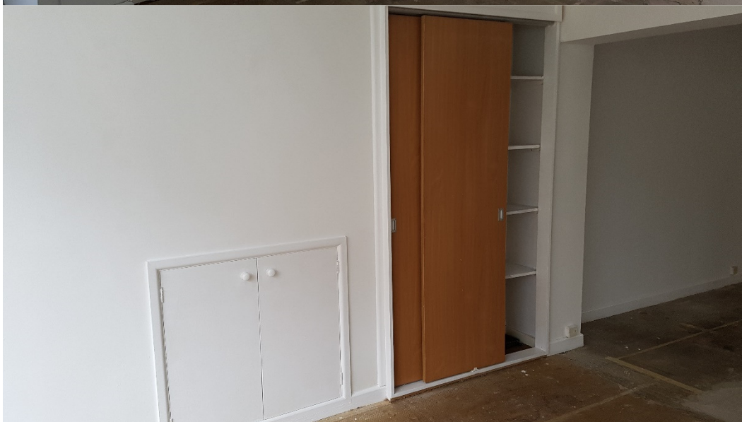
Adhoc and poorly constructed cupboards.
