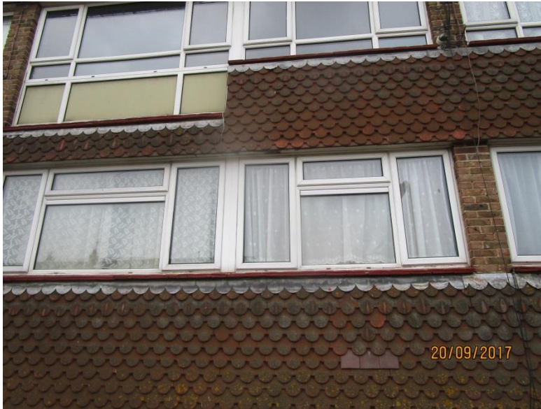
Photo 3 - Existing Facia Board and Soffit
