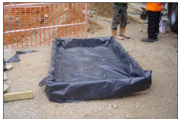
Photo 45: Soil bunding or a supporting framework covered in heavy-duty plastic sheeting is essential where there is a risk of spillages contaminating RPAs. This specifically applies to cement mixing areas and vehicle washing facilities.
