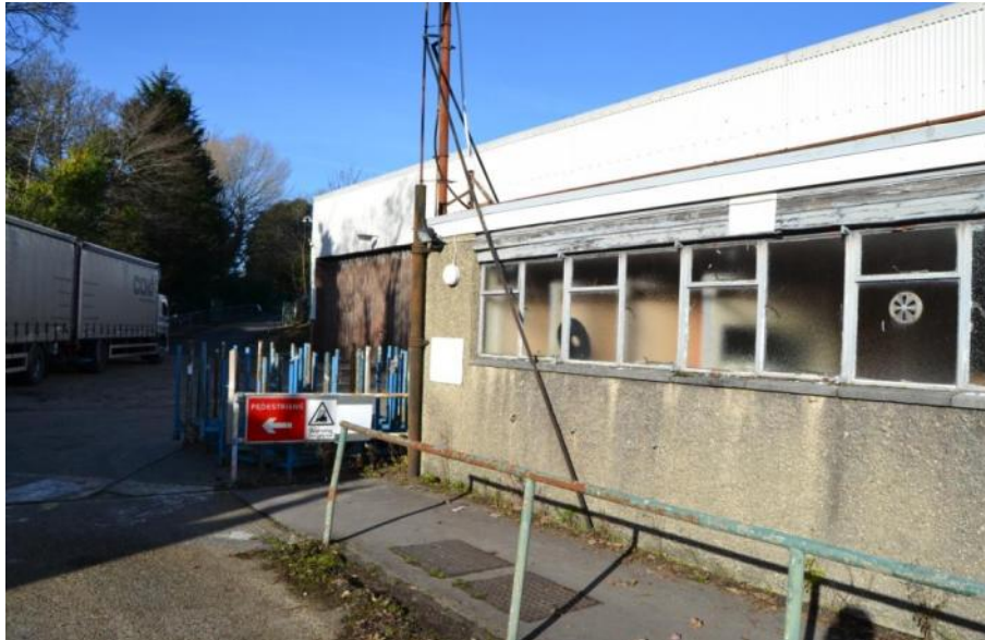
Plate 10: Southern elevation of Building 3 showing damage on the window surrounds
