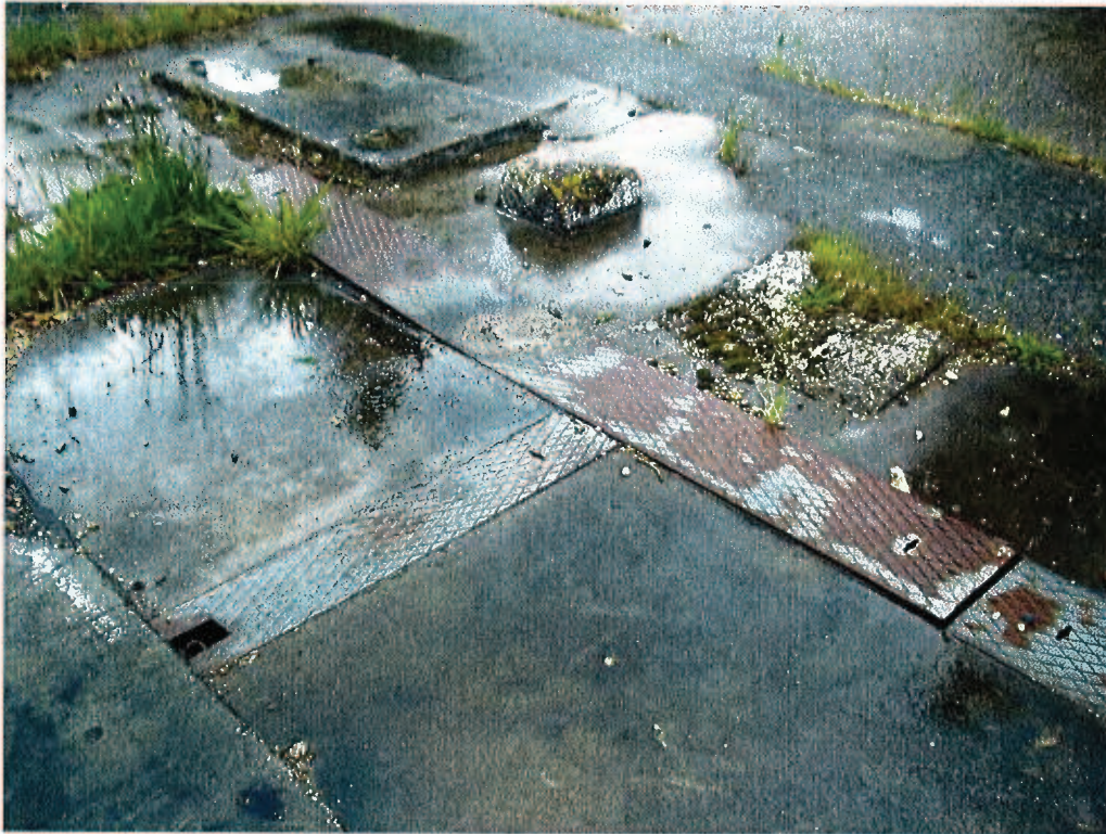
PHOTO 7 - Abandoned underground oil feeder pipework to old boiler house on location of former Scalextric factory.
