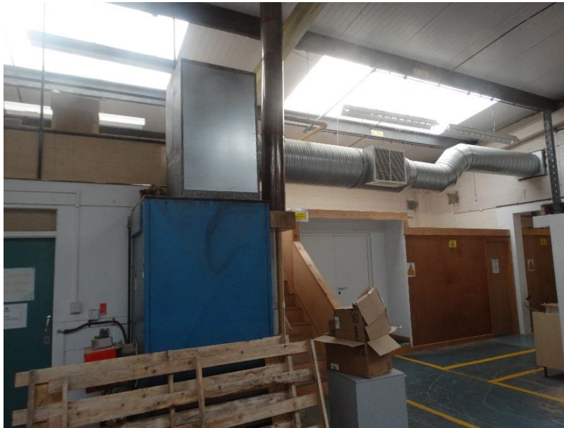
Photo 7 – additional ventilation plant within unit 1
