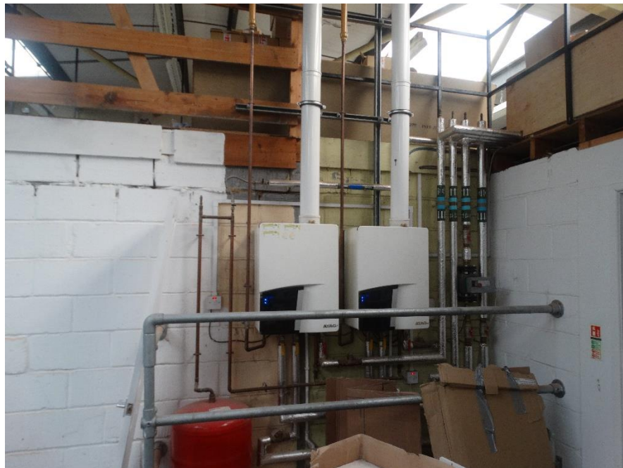
Photo 6 – showing some of the plant within unit 1.
