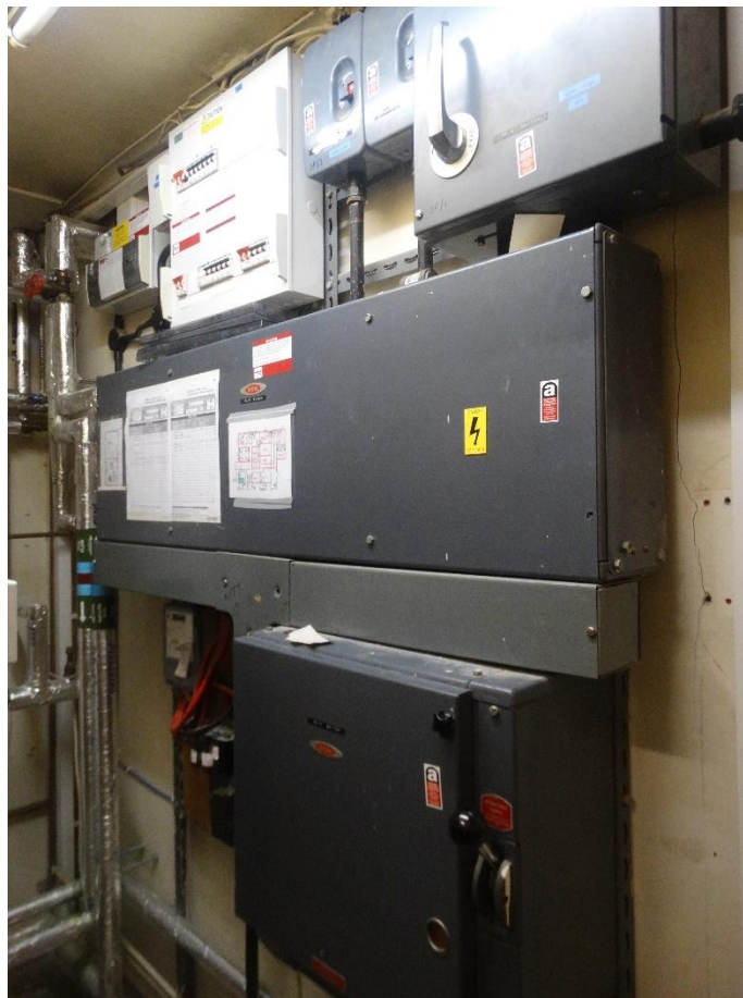
Photo 8 – Part of the power distribution network within the site (unit 1).
