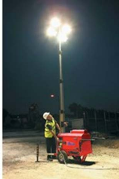
Typical Mobile Lighting Tower
