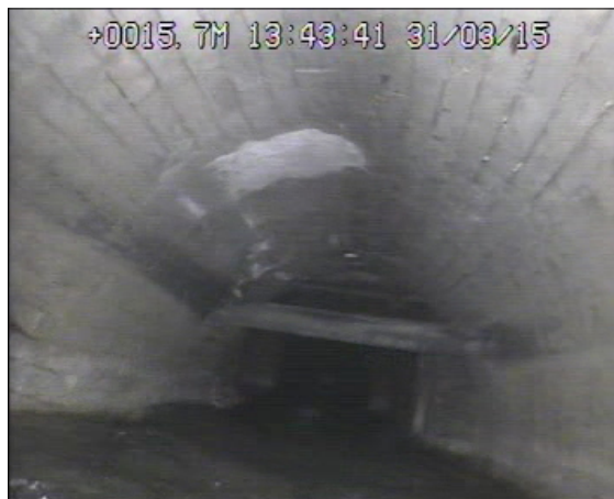
Photo: 3_9A, 00:03:28 15.7m, Displaced bricks, from 8 to 9 o'clock
