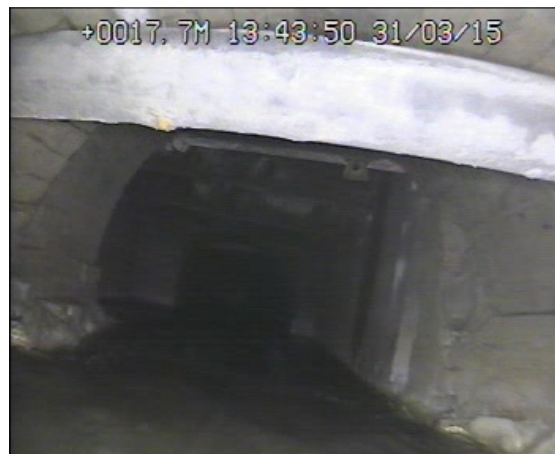
Photo: 3_10A, 00:03:36 17.7m, Other obstacles, external pipe or cable, from 10 to 2 o'clock, 10% cross-sectional area loss Remarks: SERVICE PIPE
