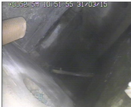
Photo: 1_12A, 00:08:10 52.5m, Connection intruding at 10 o'clock dia 225 mm intrusion 15 %
