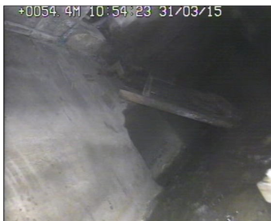
Photo: 1_15A, 00:10:21 54.4m, Junction at 09 o'clock dia 600 mm Remarks: LARGE OPEN NON RETURN FLAP VALVE WITH A BROKEN HINGE
