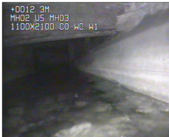
Photo: 3_7A, 00:02:08 12.3m, Other obstacles, external pipe or cable, from 10 to 2 o'clock, 10% cross-sectional area loss Remarks: SERVICE PIPE
