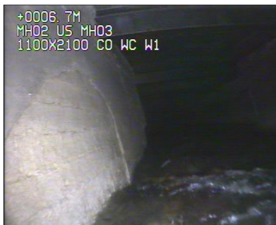
Photo: 3_5A, 00:01:38 6.7m, General remark Remarks: PATCH OF RENDER MISSING BETWEEN 7 AND 10 O'CLOCK
