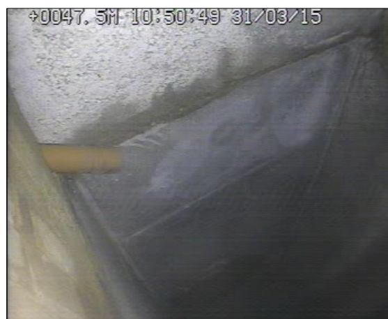
Photo: 1_11A, 00:07:03 47.5m, Connection intruding at 11 o'clock dia 100 mm intrusion 20 %
