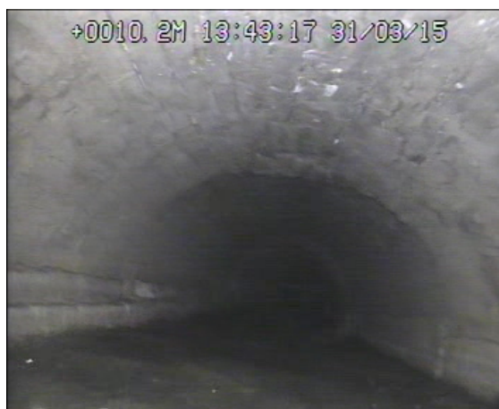
Photo: 3_3A, 00:03:03 10.2m, Missing mortar, from 8 to 9 o'clock, between 15mm and 50mm, Start
