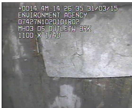
Photo: 4_6A, 00:01:32 14.4m, Other obstacles protruding through wall, from 11 to 1 o'clock, 10% cross-sectional area loss Remarks: LARGE PIECE OF CONCRETE STICKING THROUGH THE SOFFIT
