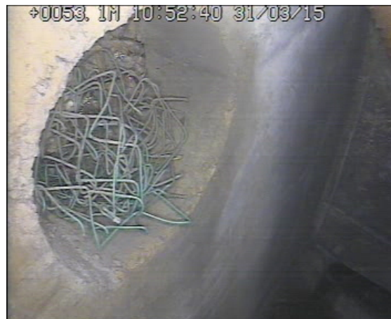
Photo: 1_13A, 00:08:39 53.1m, Junction defective, connecting pipe is blocked, at 9 o'clock, diameter 225mm
