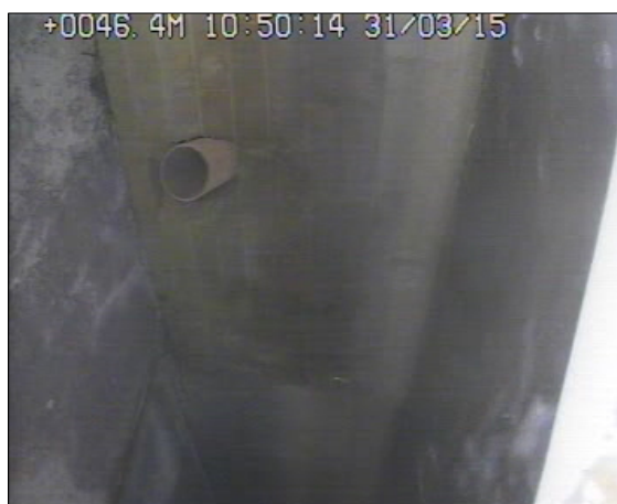
Photo: 1_10A, 00:06:16 46.4m, Connection intruding at 02 o'clock dia 150 mm intrusion 10 %
