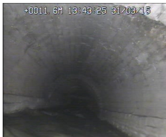
Photo: 3_4A, 00:03:11 11.6m, Missing mortar, from 3 to 4 o'clock, between 15mm and 50mm, Start
