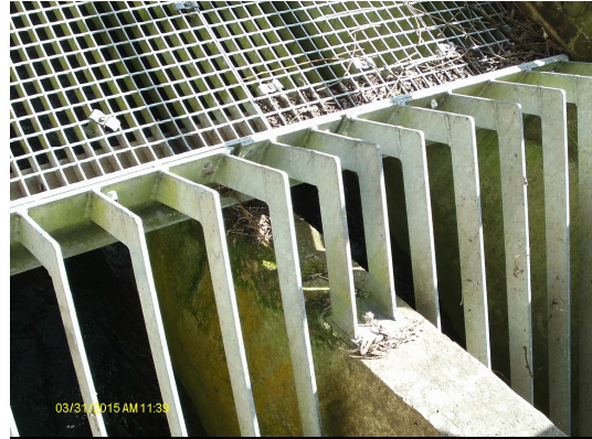
View of the Inlet trash grille
