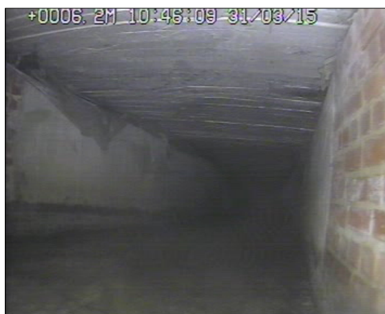
Photo: 1_6A, 00:02:08 6.2m, Line of drain/sewer deviates right
