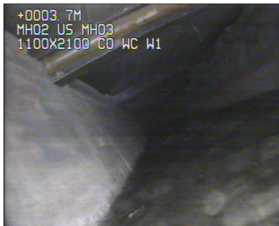
Photo: 3_3A, 00:00:22 3.7m, Other obstacles, external pipe or cable, from 10 to 2 o'clock, 5% cross-sectional area loss Remarks: SERVICE PIPE
