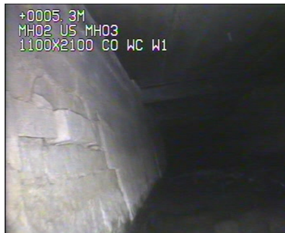
Photo: 3_4A, 00:00:30 5.3m, Displaced bricks, at 3 o'clock Remarks: APPEARS TO BE AN OLD BLOCKED OFF JUNCTION
