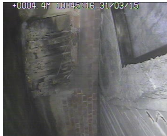
Photo: 1_5A, 00:00:11 4.4m, General remark Remarks: OLD INLET ACCESS COVER
