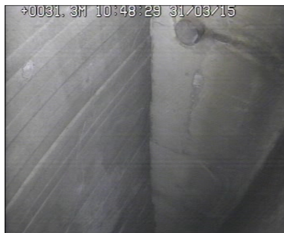
Photo: 1_9A, 00:04:28 31.3m, Connection intruding at 02 o'clock dia 100 mm intrusion 5 %
