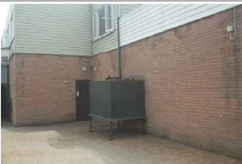
Oil tank adjacent to north of central complex building and which supplies the heater for the indoor swimming pool. Note the pipework from the oil fill point routed to the tank over the roof of the building.
