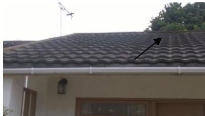
Plate 4.3: Gaps under ridge tiles
