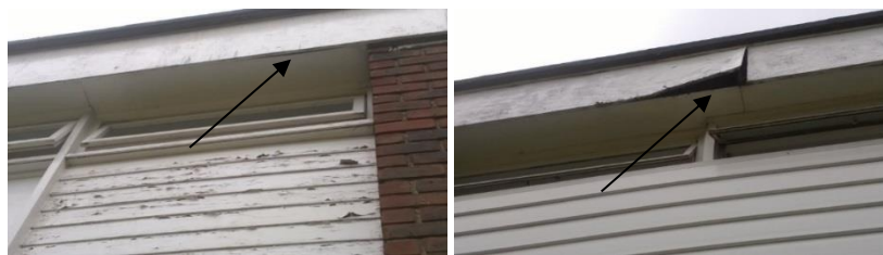
Plate 4.8: Gaps within the timber soffit boxes (Buildings 5 & 29)
