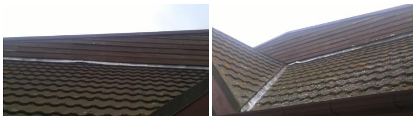
Plate 4.15: The western gable end of Building 10 had lifted lead flashing and lifted cladding
