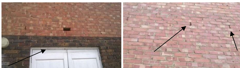
Plate 4.10: Weep holes and missing bricks within the chimney breast of Building 41
