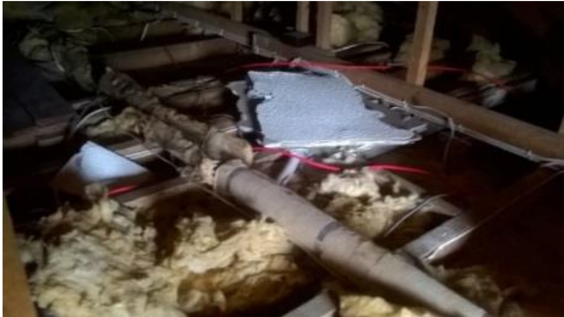
Plate 4.6: A large number of exposed cables were present preventing safe access
