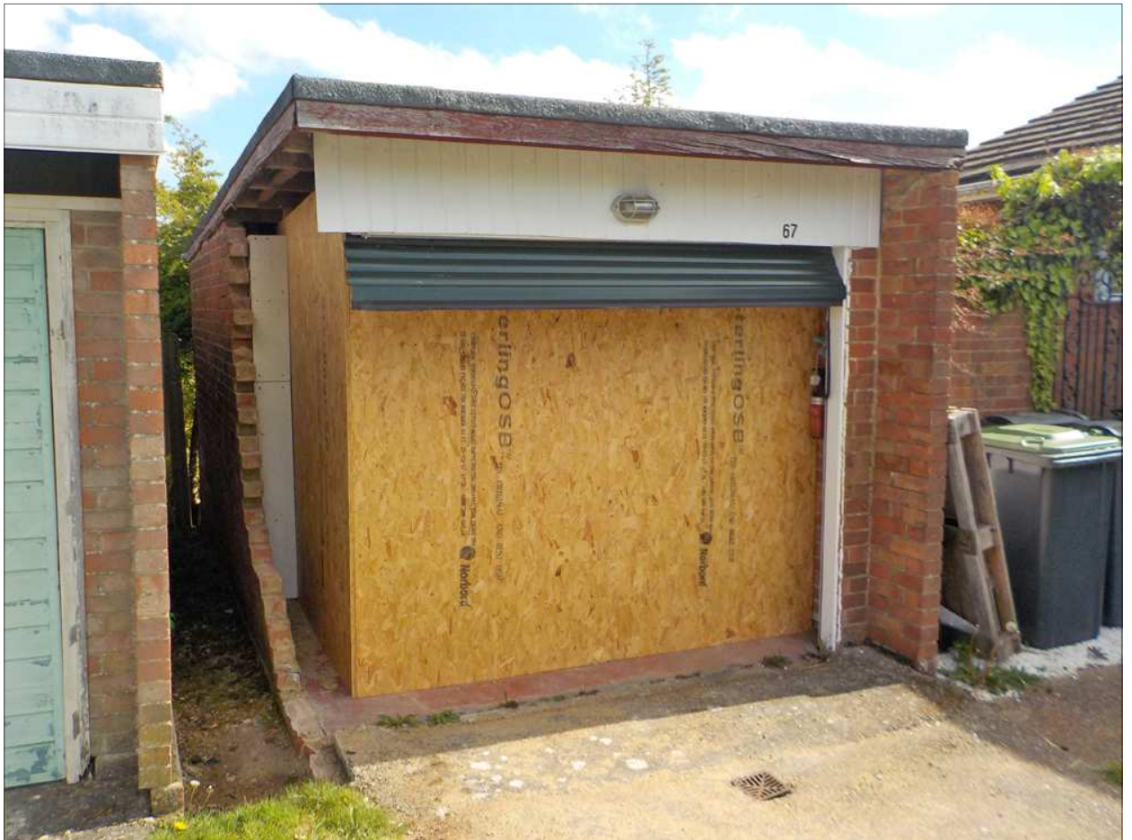
Damage to the garages (both No.'s 67 & 67)
