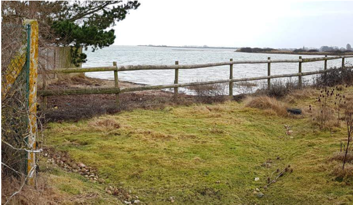
Fig 3.5.3 – Photograph showing French drain outfall
