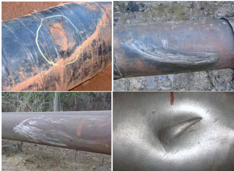
Figure 24. Examples of Severe Damage to Pipelines
