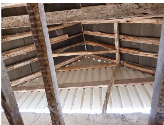
Figure 9 - Roof structure to be re-built
