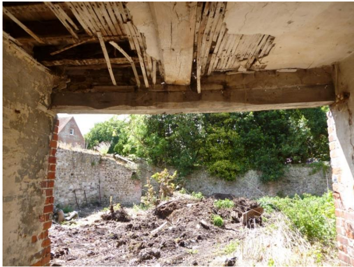
Figure 24 – Lintel that needs structural assessment
