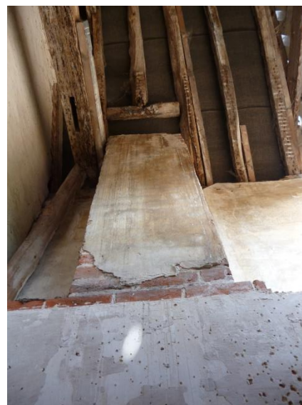
Figure 40 – Chimney flue. Lime mortar plaster to be removed
