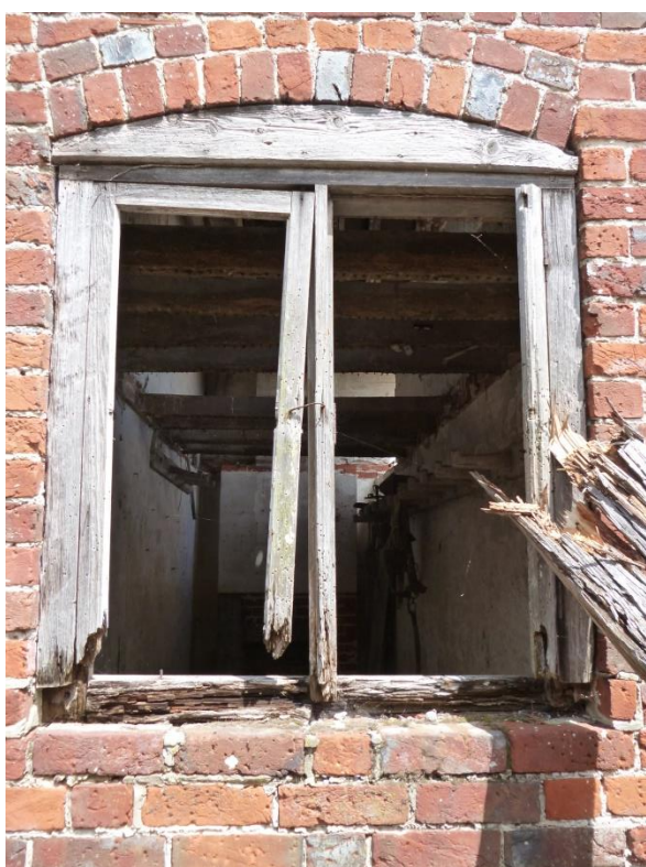
Figure 20 – derelict casement window
