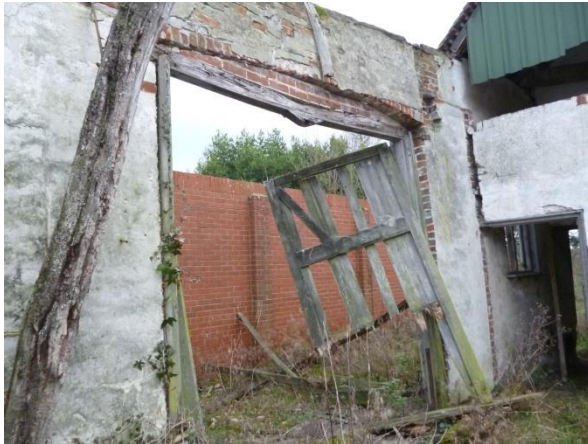
Figure 3 – Semi derelict archway with loosely hanging doors panels
