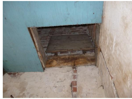
Figure 27 – Hatch to attic to be covered
