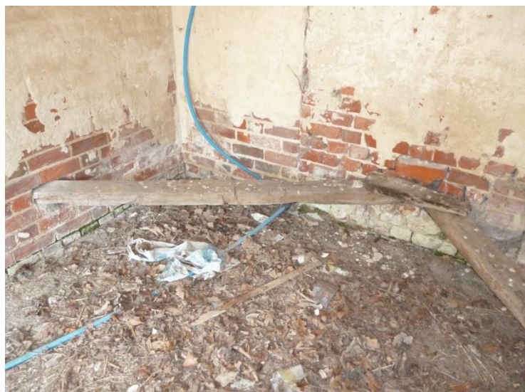
Figure 38 – Wooden structure inset in brick walls to be removed.
