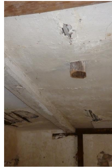
Figure 25 – Post in need of removal
