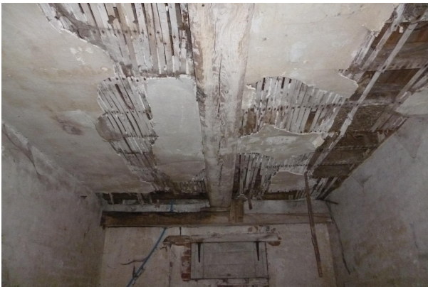
Fig. 1 - chamfered beams. Dilapidated plaster and lath finish.
