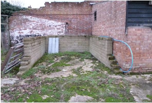
Fig. 2 - walling of blockwork laid flat
