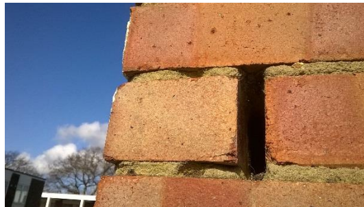
Plate 6: Weep Hole in Building 46
