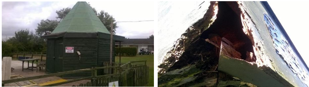
Plate 1: Gap in Soffit of Building 1
