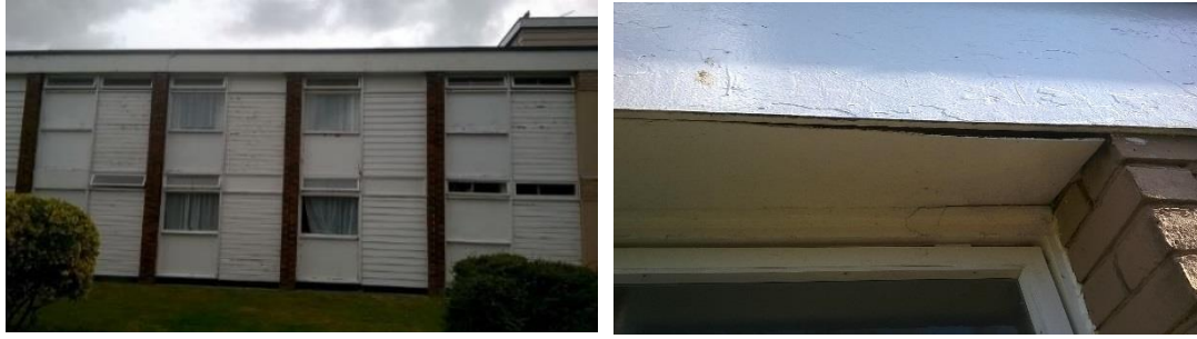
Plate 3: Gap in Soffit of Building 5
