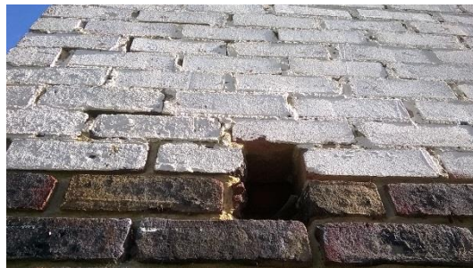
Plate 7: Gaps in Brick Chimney of Building 46 Left by Missing Bricks
