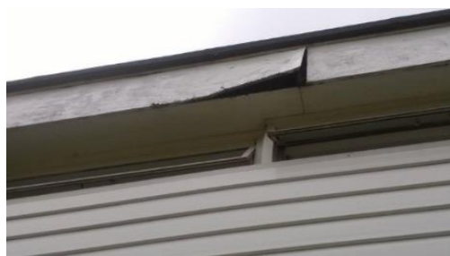
Plate 5: Gap in Soffit of Building 29
