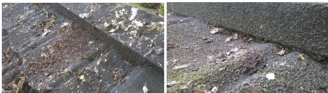
Plate 2: Gaps Under the Ridge Tiles Were Blocked With Dirt and Moss
