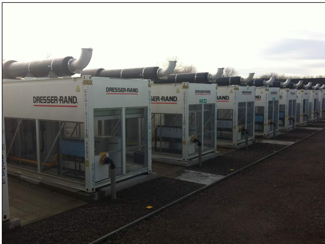
Figure 5 Typical Containerized generator
