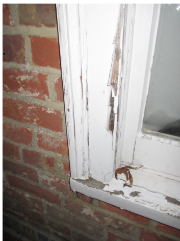
Fig 4 – Photo of typical timber window condition
