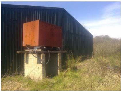
Photograph 8 (P8) Above ground fuel tank in the centre of the study area.
