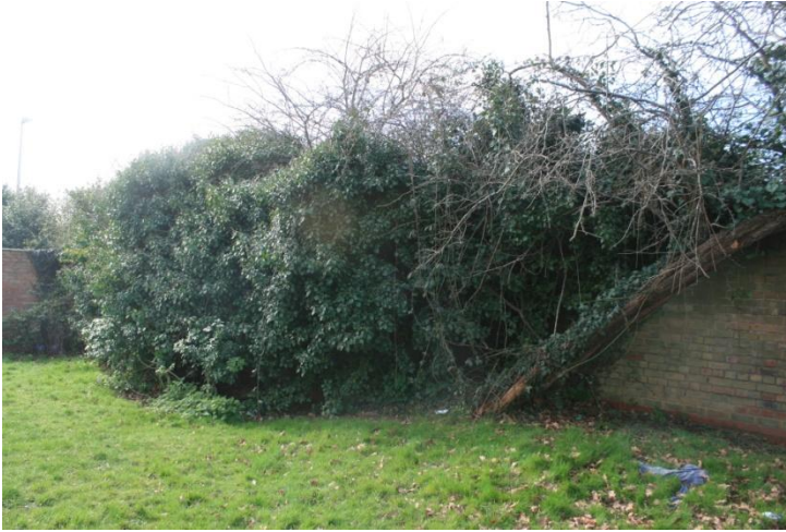
Photograph 5: Southern wall with dense ivy
