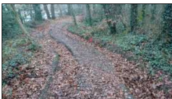
Site photo 1: Showing deep rutting on existing byway.
