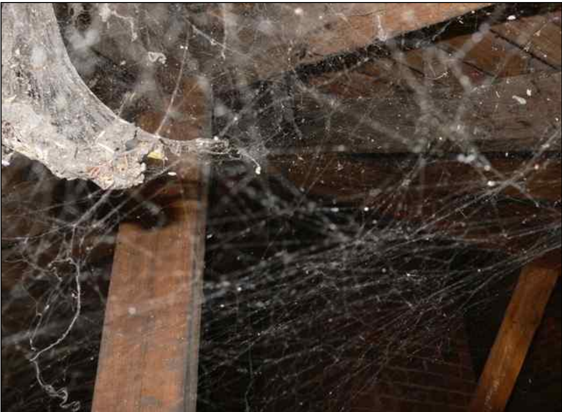
Photo 17 The upper roof had an accumulation of cobwebs again indicating lack of recent bat use.
