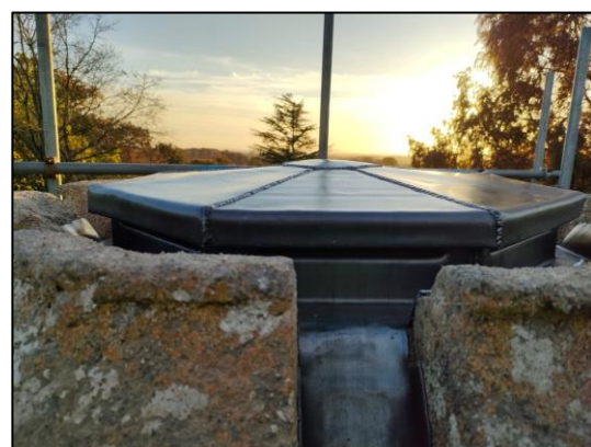
Photo 23 Ventilation feature in capping – approximately 200 x 20mm
