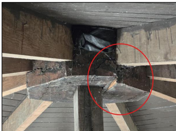
Photo 9 Split timber at central octagonal roof plate
