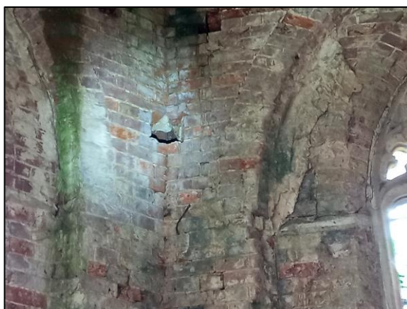
Photo 11 Missing and crumbled brickwork in interior
