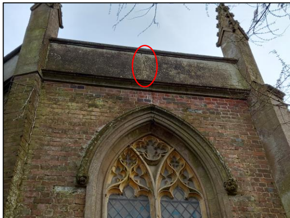
Photo 15 Exterior showing brickwork and render sections and crack at upper level
