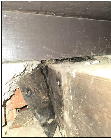
Photo 7 Bricks removed to inspect beam decay
