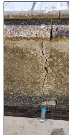
Photo 16 Crack in high level masonry for repair – Face 2
