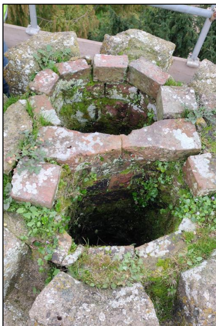
Photo 20 View of uncapped chimney
