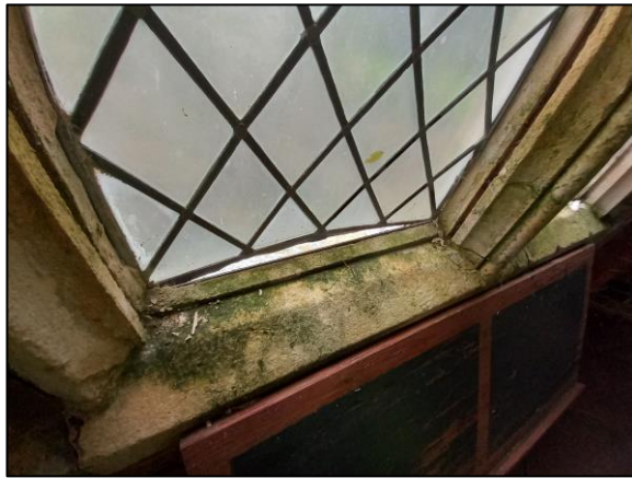
Photo 13 Interior image of gap to bottom of window
