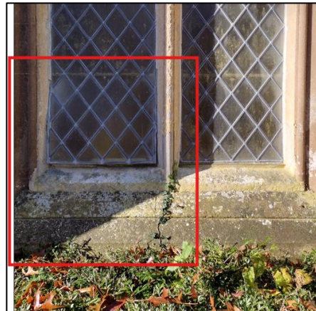
Photo 14 Exterior image of gap to bottom of window.
