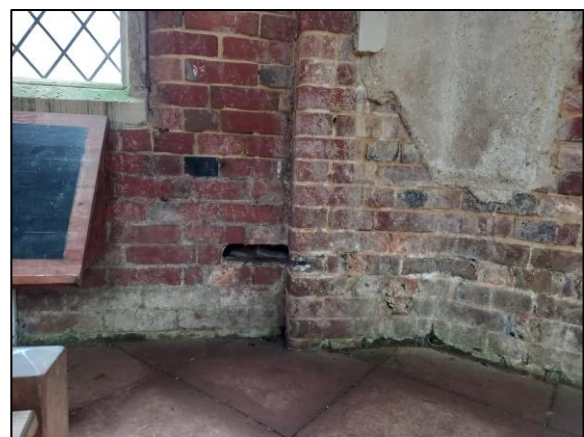
Photo 12 Missing bricks in interior wall
