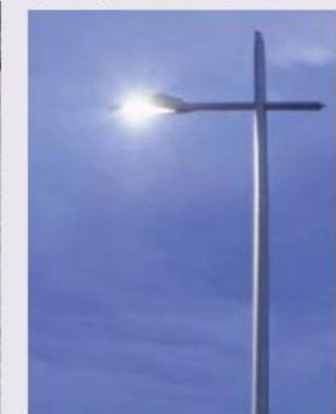
Street lighting - columns
