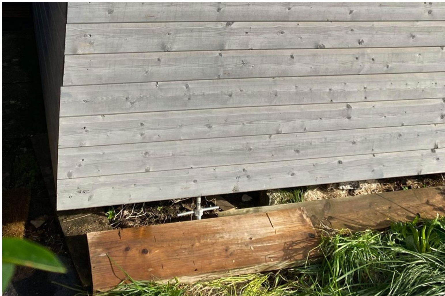
Metal jack supports for level siting visible, mobile home not attached to the ground.
