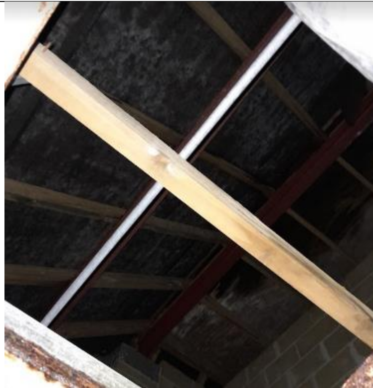
Figure 13 - View of northern internal loft cavity through corroded hole in ceiling of toilet block.
