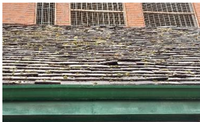
Figure 11 - View of lifted tiles on the toilet block.
