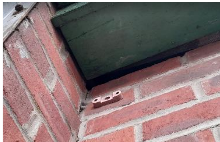
Figure 12 - View of gap beneath soffit to the south of the toilet block.
