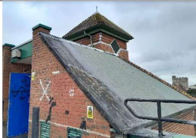
Figure 8 - View of the northeastern tower showing gaps beneath lead flashing and area of tiled roof.
