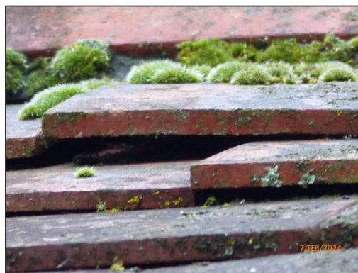
Figure 18: Raised roof tile leading to void between tile and felt underlay.
