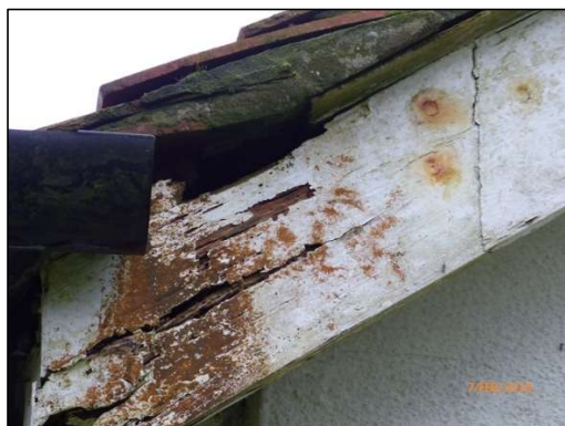
Figure 17: Rotten soffit on south-east corner.
