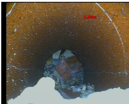
Observation [4]: End Point: redundant
