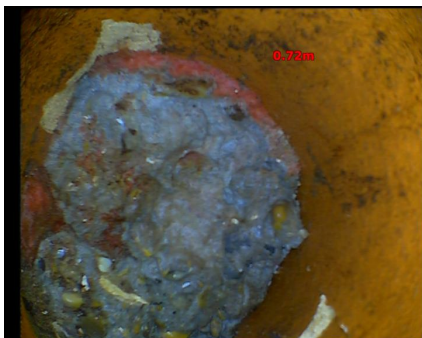
Observation [4]: concreted redundant pipe
