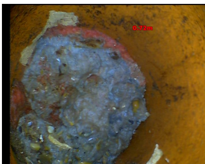
Observation [5]: End Point: redundant
