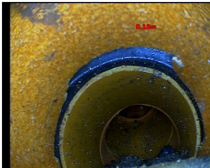
Observation [3]: damaged plastic to clay pipe
