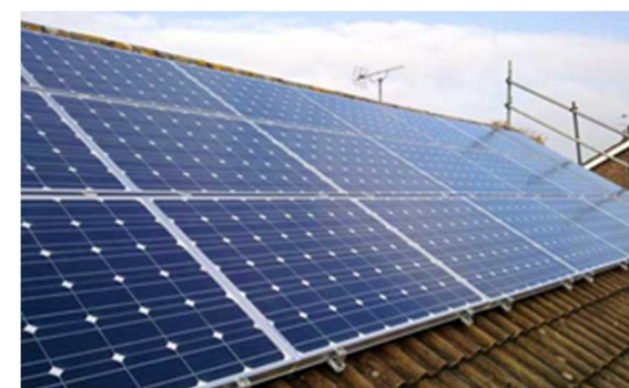
Picture 1 —Roof mounted PV panels
