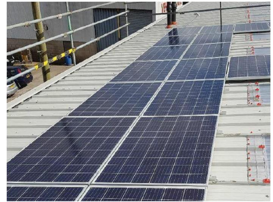
Roof mounted PVs
