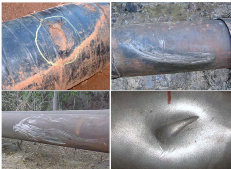
Figure 24. Examples of Severe Damage to Pipelines
