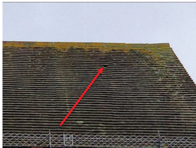
Figure 11. View of a broken concrete tile.
