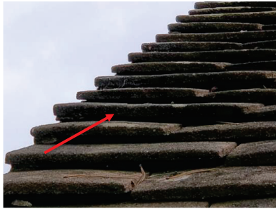
Figure 10. View of the gaps present underneath the concrete tiles.
