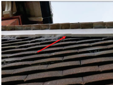
Figure 12. View of the gaps underneath the fascia board by the hanging tiles.
