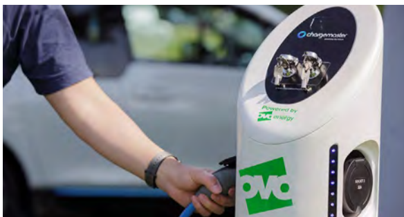
Public electric car charging points incorporated into the development
