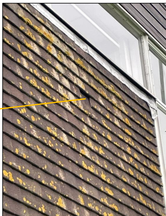
Photos 15 and 16 PRF E – missing hanging tile on east elevation of two-storey section of building.
