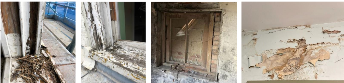
Fig. 09- Left to right: Existing 1 st floor windows to front elevation ; Existing party wall treatment to southeast boundary; Example of water damage in the first floor office 'B'.
