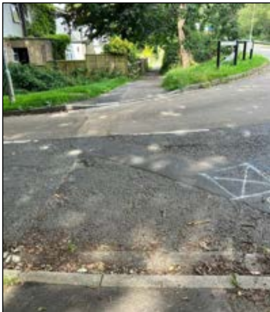
Photograph 61: Dropped Kerb crossing at Jackdaw Close
