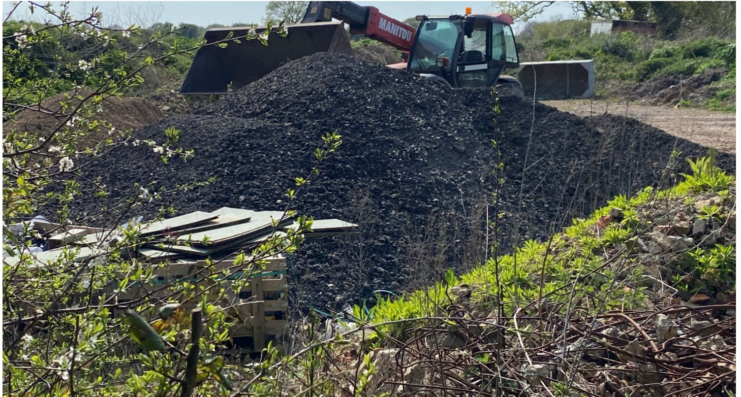
Fig 16: The area of the SAM that is being used for storage of builder's waste (old pallets and twisted metal and concrete can be seen in the foreground) and a quantity of recycled tarmac road planings.
