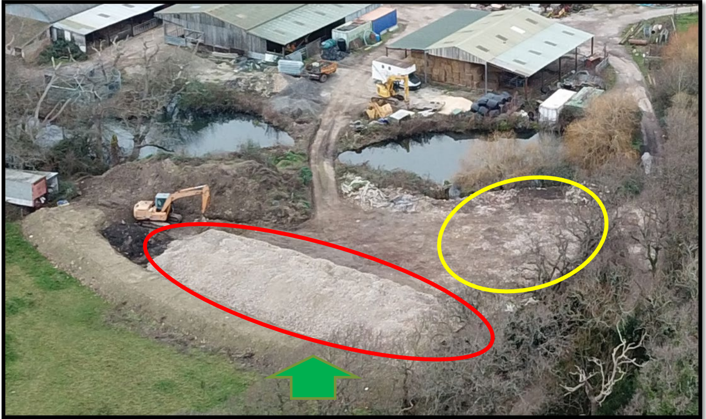
Fig 15: Drone photograph of unconsented (HBC), unpermitted (Environment Agency) mixed builders waste & burning Tip at Tournerbury Farm. The mixed builders waste which has been crushed in between Christmas and New Year (when local authority and Environment Agency staff are on holiday) can be seen (red oval) and the waste dumping area is now clear (yellow oval). The activities in this area are screened by an unconsented earth bund along the southern boundary which sits on top of the SAM at its eastern end (green arrow).
