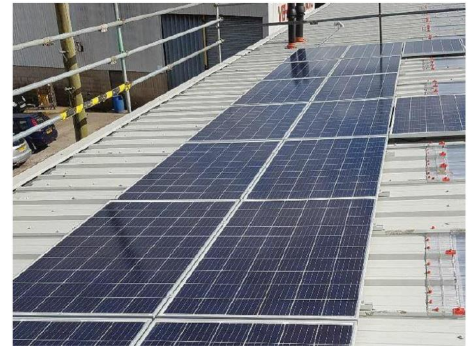
Roof mounted PVs
