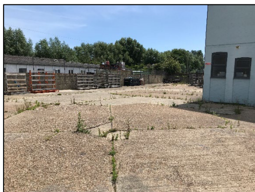
Figure 2: Vegetation present within the cracks
