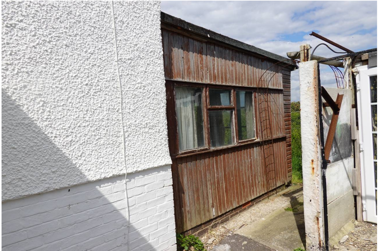
Photo 11 – View of rear addition to No. 25 with the dilapidated garage seen on the right.
