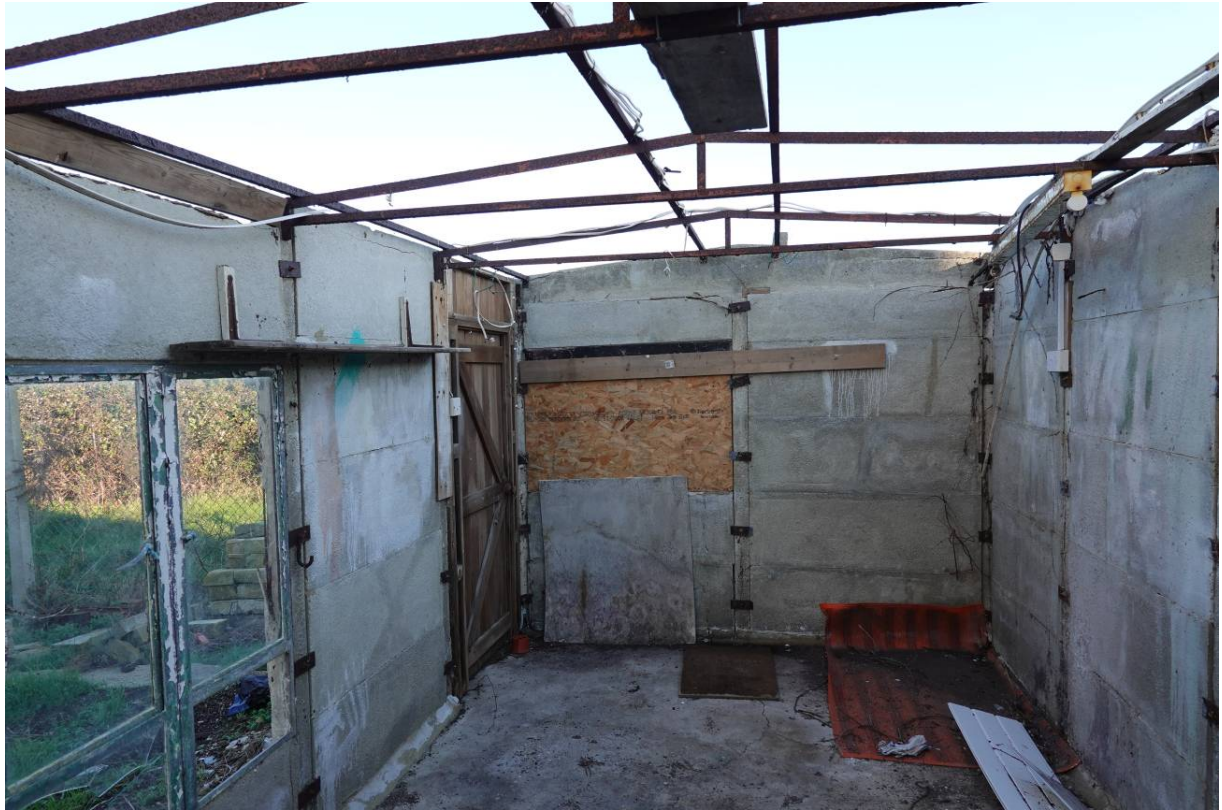
Photo 18 - View inside the dilapidated garage after the roof was removed some months earlier.
