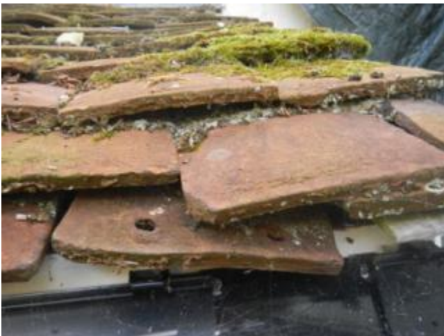
Detail of lifted tile
