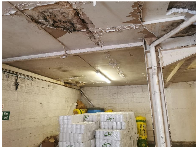
Inside of building southern facing- showing internal cracks and mould
