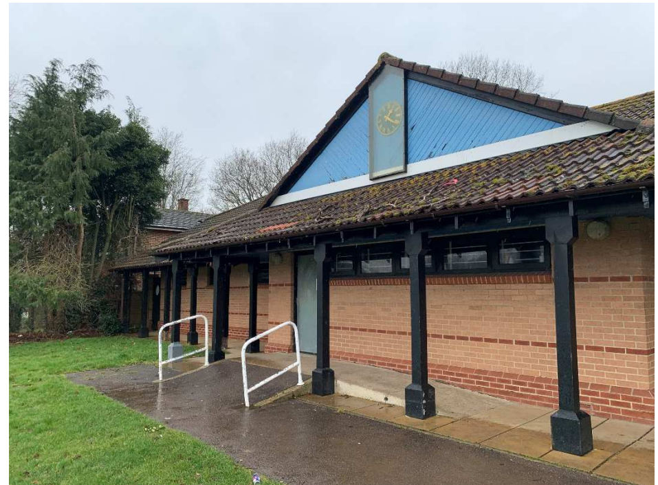
Existing South Elevation with non-compliant DDA ramp access
