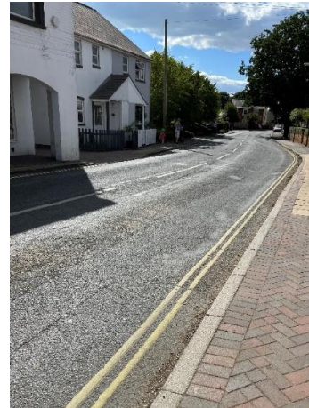
Photograph 4: Station Road conditions
