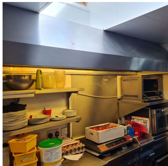
Fryer Extract – to be removed.
