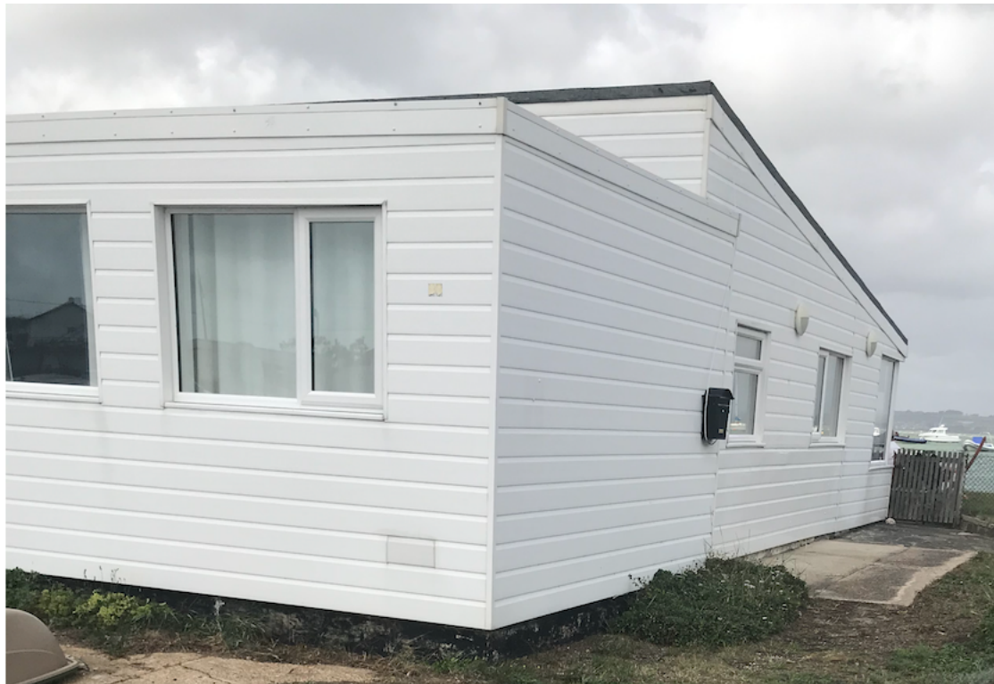
Photo 1: Looking south, original cladding showing poor quality of installation, repairs, and dis-colouration
