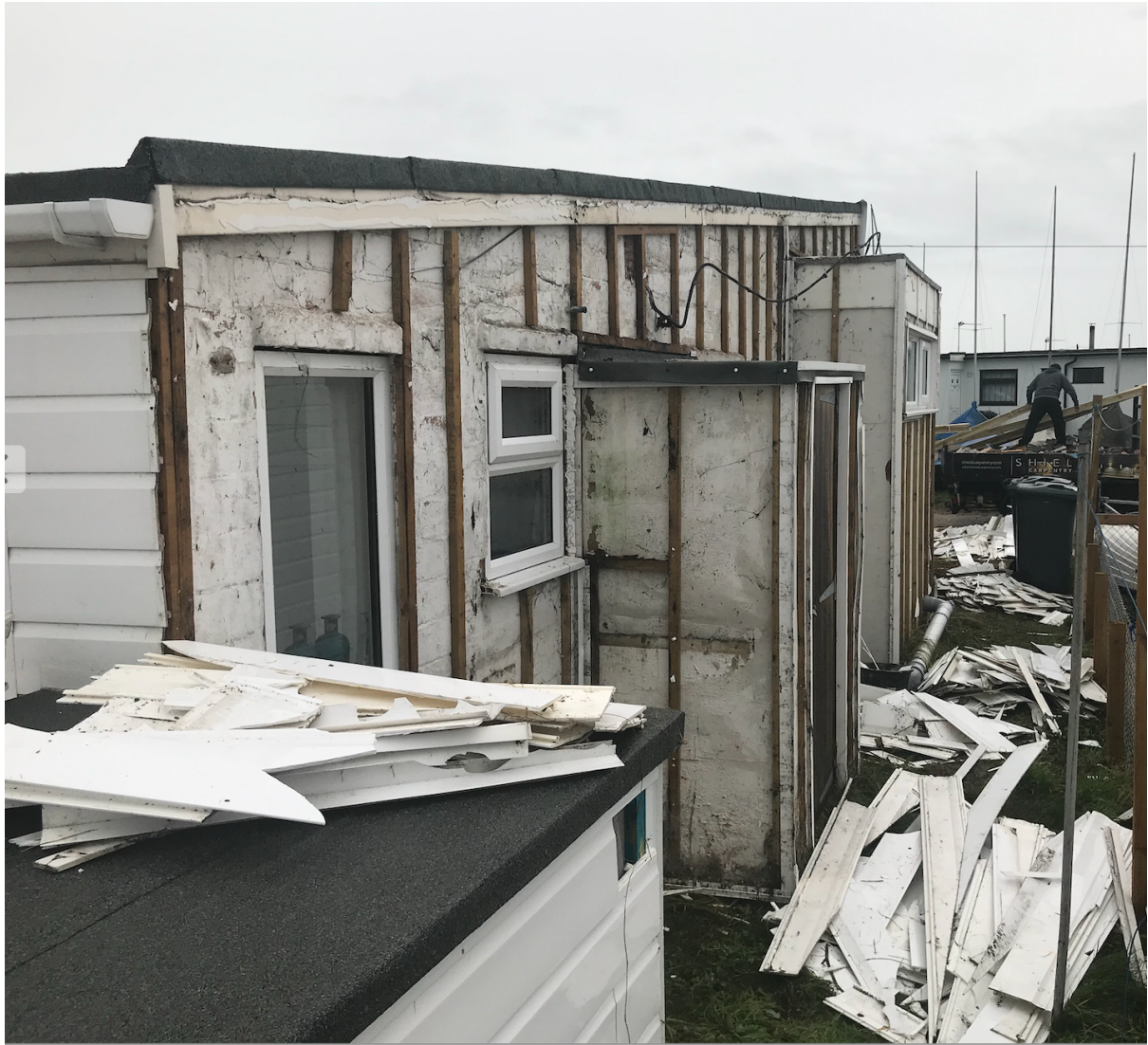
Photo 2: West elevation showing original brickwork and old battens, lack of membrane and state of the original cladding as it was removed.
