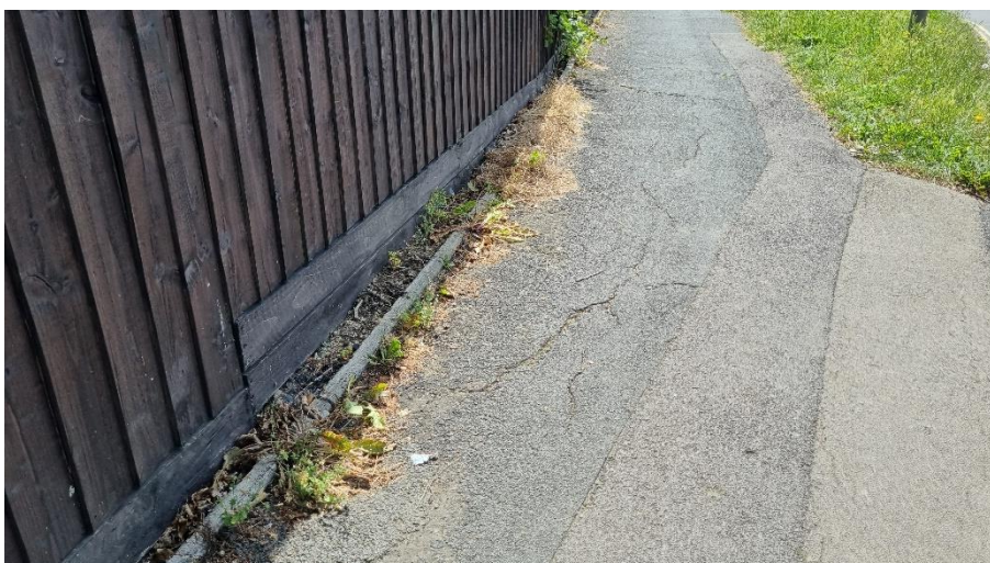
Photo 47: Poor footway surface on Langstone Road (near Woodbury Avenue)
