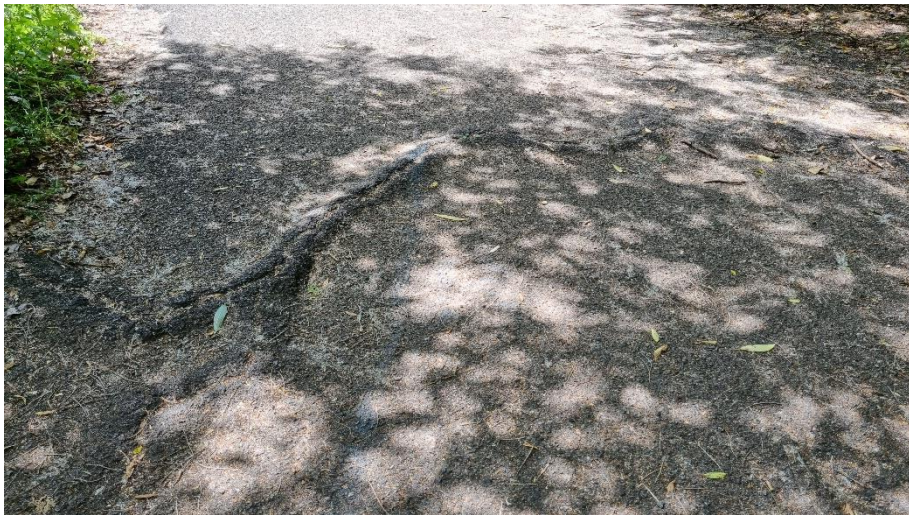
Photo 41: Damaged surface on pedestrian / cycle path north of development site
