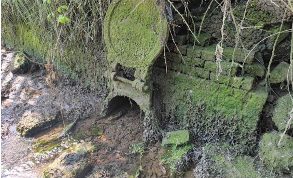
Figure 5 – Main River outlet partially blocked
