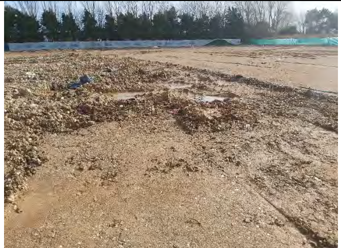
General view looking to northeast corner. Poned water following wet weather and storms on sacrificial layer.
