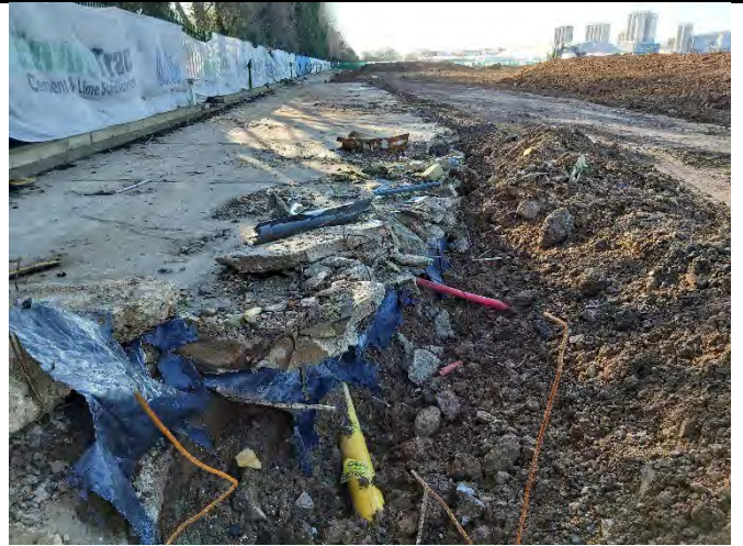
Excavation extent along northern boundary incomplete. Gas main present.
