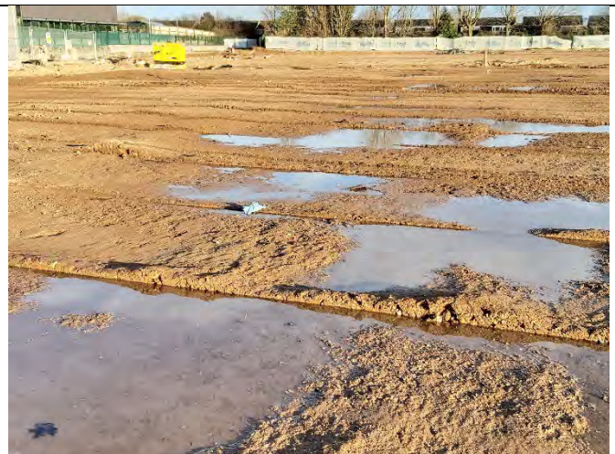
Ponded water on top of formation sacrificial layer.
