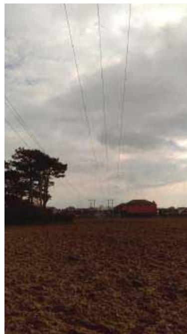
Photo 3: OH powerlines running across site
